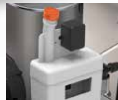
Water tank with anti-scale device
